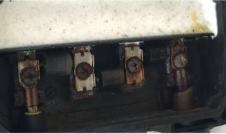
Resulting corrosion after 3 years near coast
